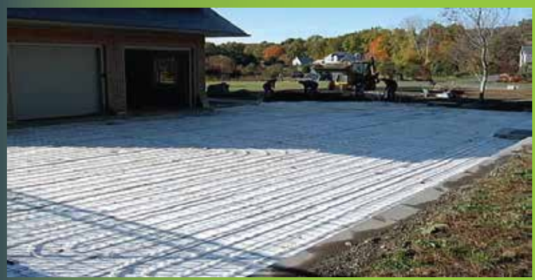
Snow Melt System Before
