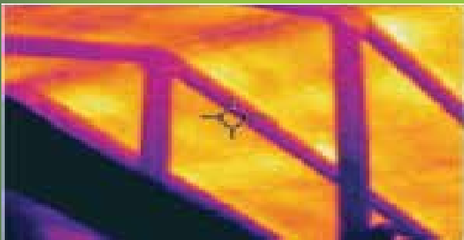
Thermal imaging of an attic without ThermaSheet® roofing underlayment. Temperature is 129°
