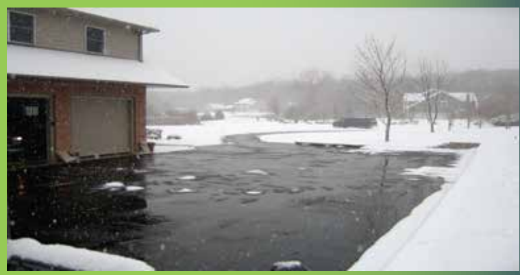
Snow Melt System After
